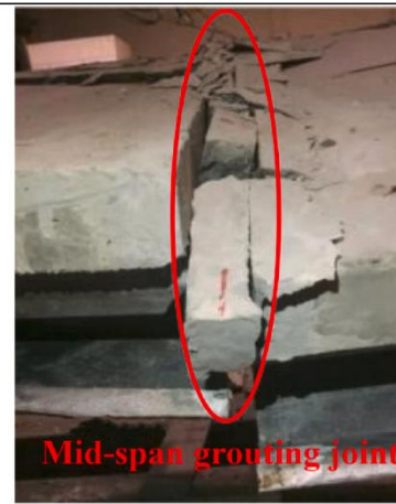
(d) Destruction of mid-span grouting joint (PG1 and PG2)
