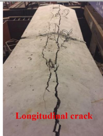
(c) Longitudinal crack in PG1 and PG2
