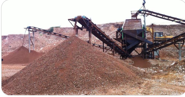
On-site Pre-screening Treatment
